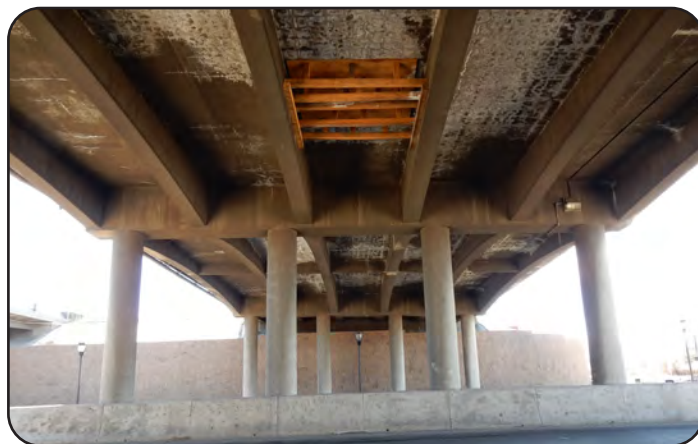
Image 2. Severe Deck Deterioration on I-70 WBND over West 32nd (E-16-HF)
