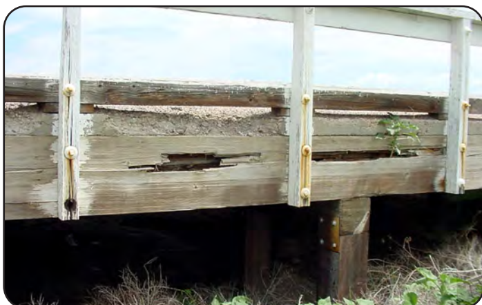
Image 4. Rotting Girder on US 36 ML over Draw (F-19-E)
