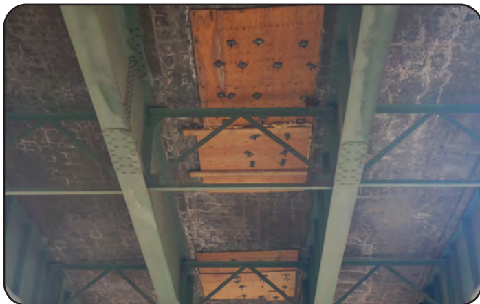
Image 11. Severe Deck Deterioration on I-270 WBND over SH265, UPRR, BNSF RR (E-17-IH)
