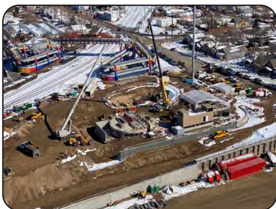
Image 16. Aerial of Pump Station near York Street
