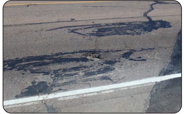
Image 6. Potholes and Settling on I-25 NBND over Academy Blvd (I-17-GQ)
