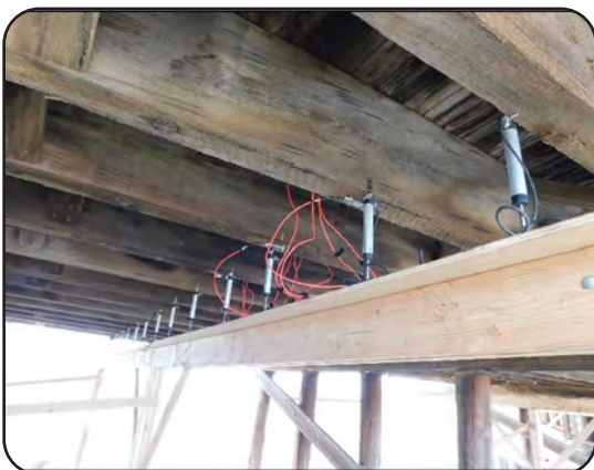
Image 22. Load Testing Sensors Measuring Displacement on US 36 over Vega Creek in Washington County
